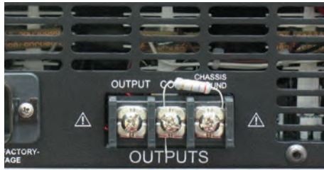
Figure B.2.38 – Output Terminal Resistor Location
